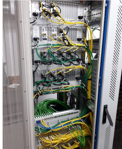
Rack in the serverroom
