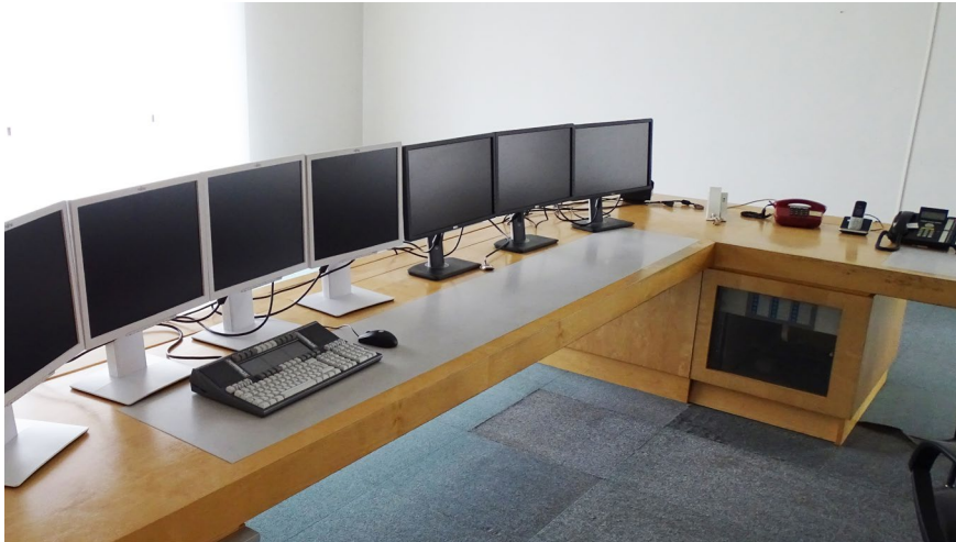
Emergency Control Center
