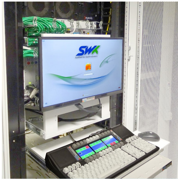
System room with control panel
