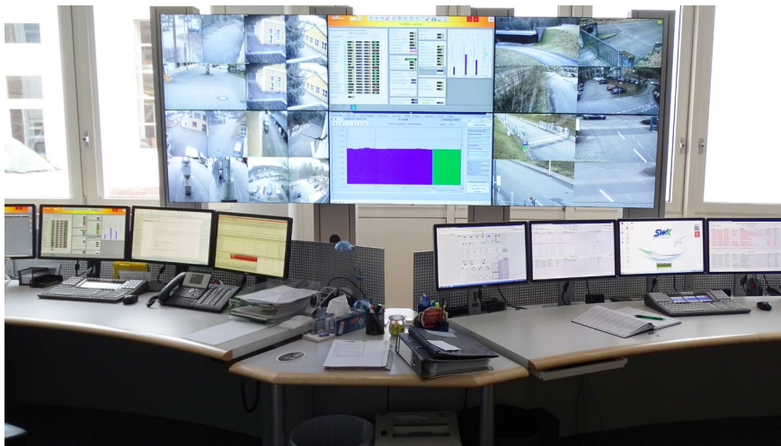
Multi-utility control center
